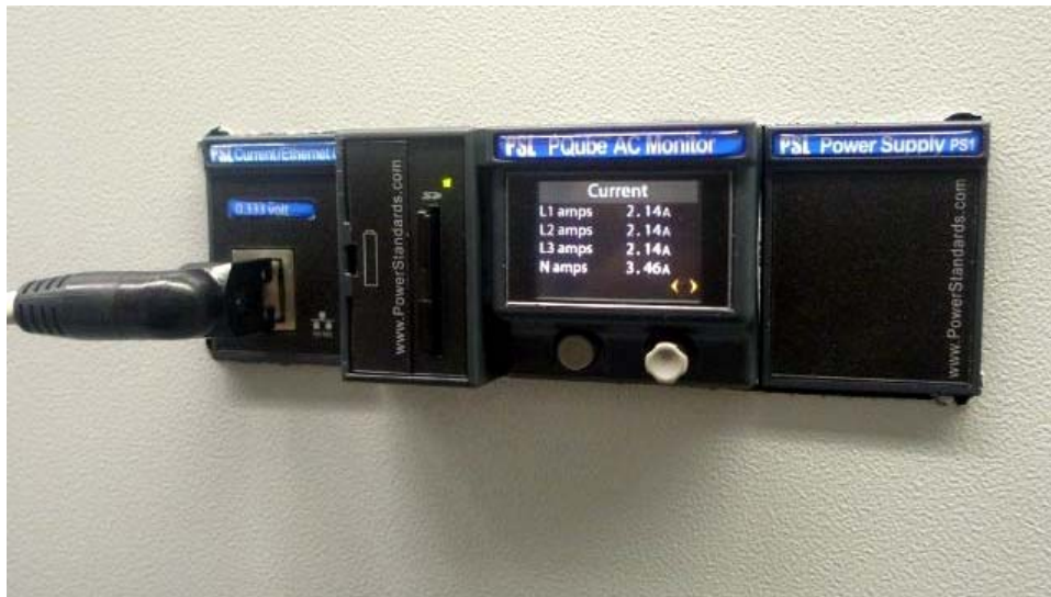
Foto 2 - Sample Caption - PQube installation at sample customer
