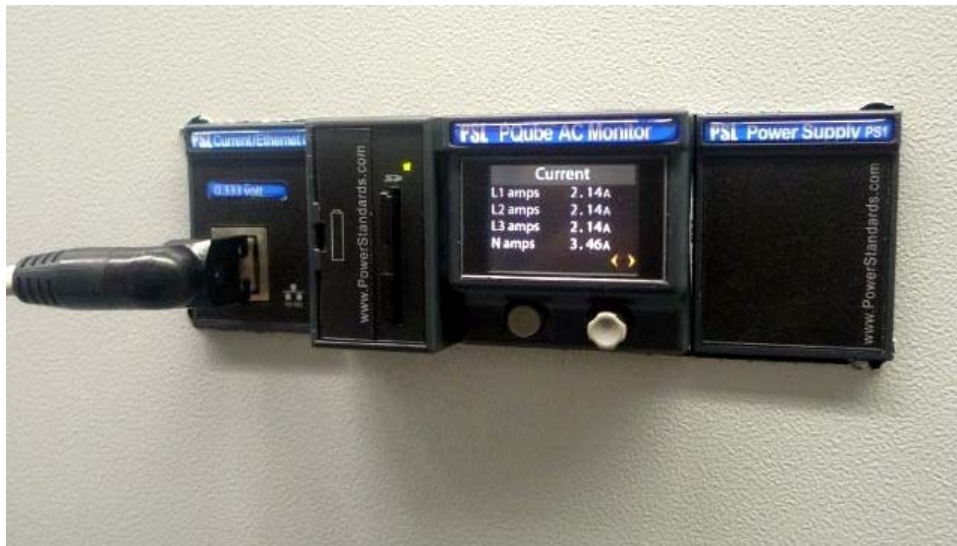
Foto 2 - Sample Caption - PQube installation at sample customer
