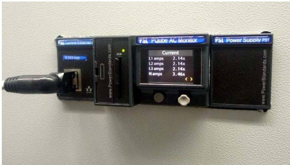
Photo 2 - Sample Caption - PQube installation at sample customer
